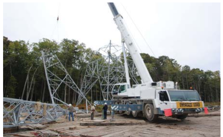
One of MYR's new 200T A T cranes helps to set one of the new lattice towers along the Carson to Suffolk 500kV transmission line.
