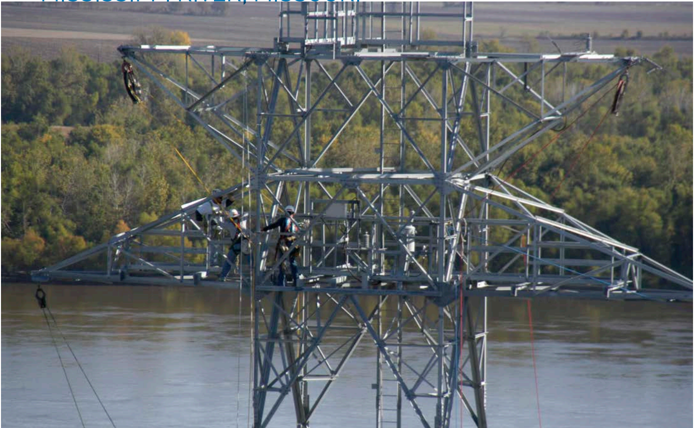
A crew at work on one of the 400' structures overlooking the Mississippi River near Festus, MO
