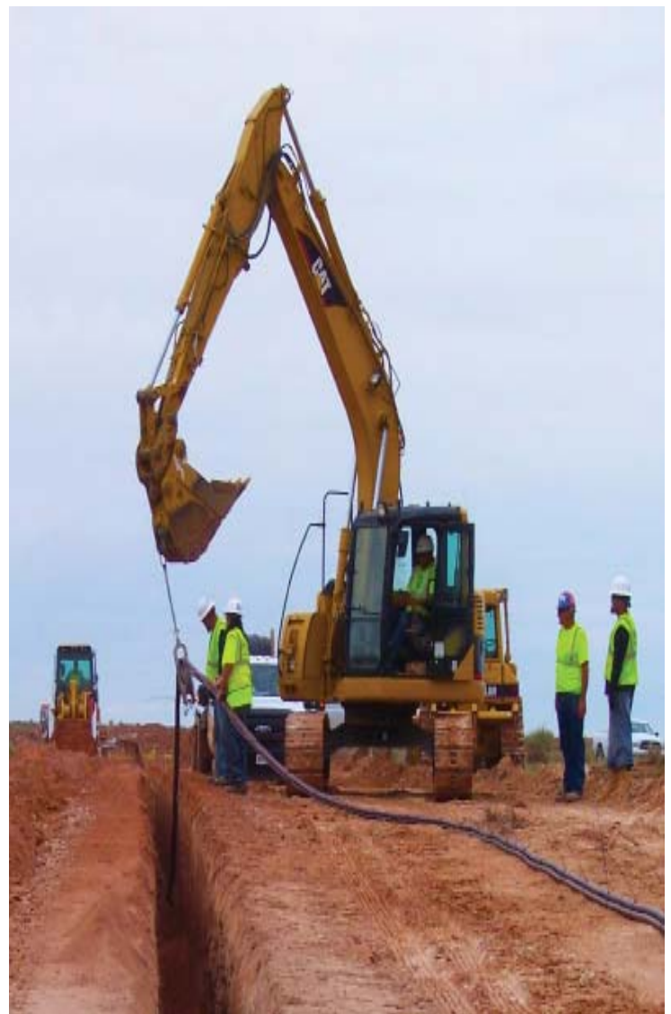
Crews overseeing trench placement of the 3-phase cable for the Dry Lake II Wind Farm collection field.
