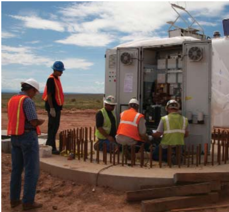
L to R: Howard Filleman, Lalis Garcia, Justin Riley, Mike Brice and Sam Lable of Sturgeon observe and conduct conductor terminations
